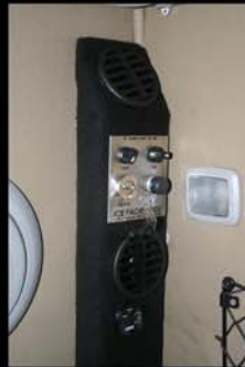
DUCTED VENT POSTS
